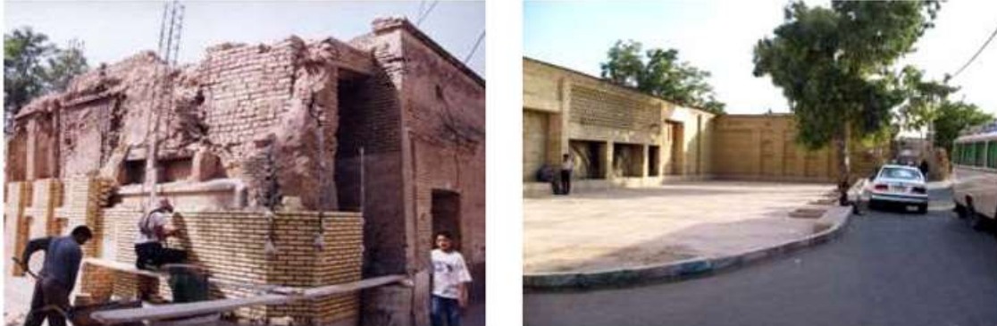
Figure 9 Physical rehabilitation of Sang-e Sia axis and newly constructed open space in front of the Bibi-dokhtaran shrine
